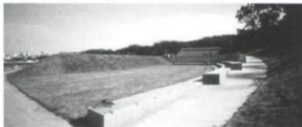
Figure 4. The West Bluff picnic area at Crissy Field was built with earth excavated to restore wetlands. (Photograph by M. Boland)
