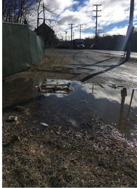
Photograph 25. Depression filled with water, south west parking area, Photo Taken April 1, 2017.
