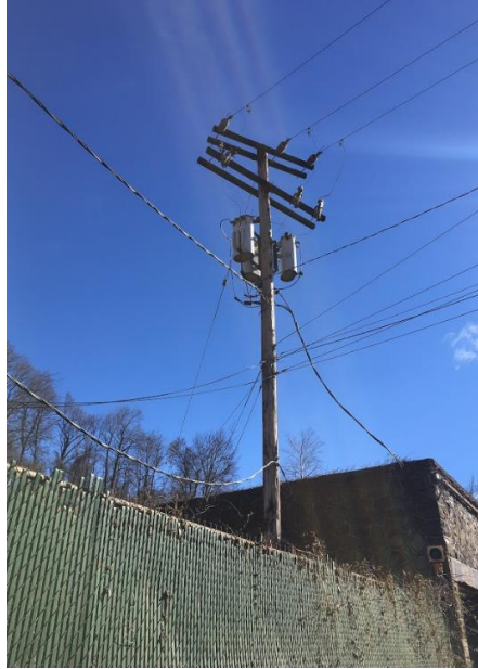
Photograph 15. Transformer on telephone pole, Building 3 pictured, Photo Taken April 1, 2017.
