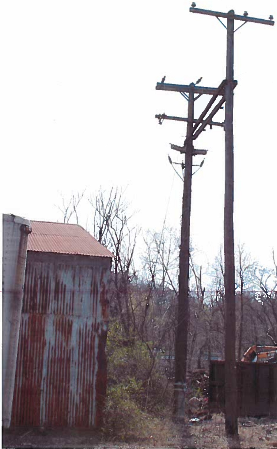
Figure C.2.11: Old Transformer Location (Identified as Concern 10)
