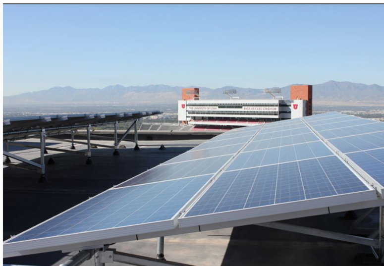
Figure 3: Two of the solar arrays on the west penthouse of the J. Willard Marriott Library, University of Utah. Source: https://unews.utah.edu/red-goes-for-green-energy/
