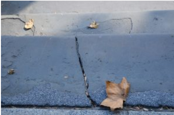
Figure 1: Regular cracking in steps and pathway
