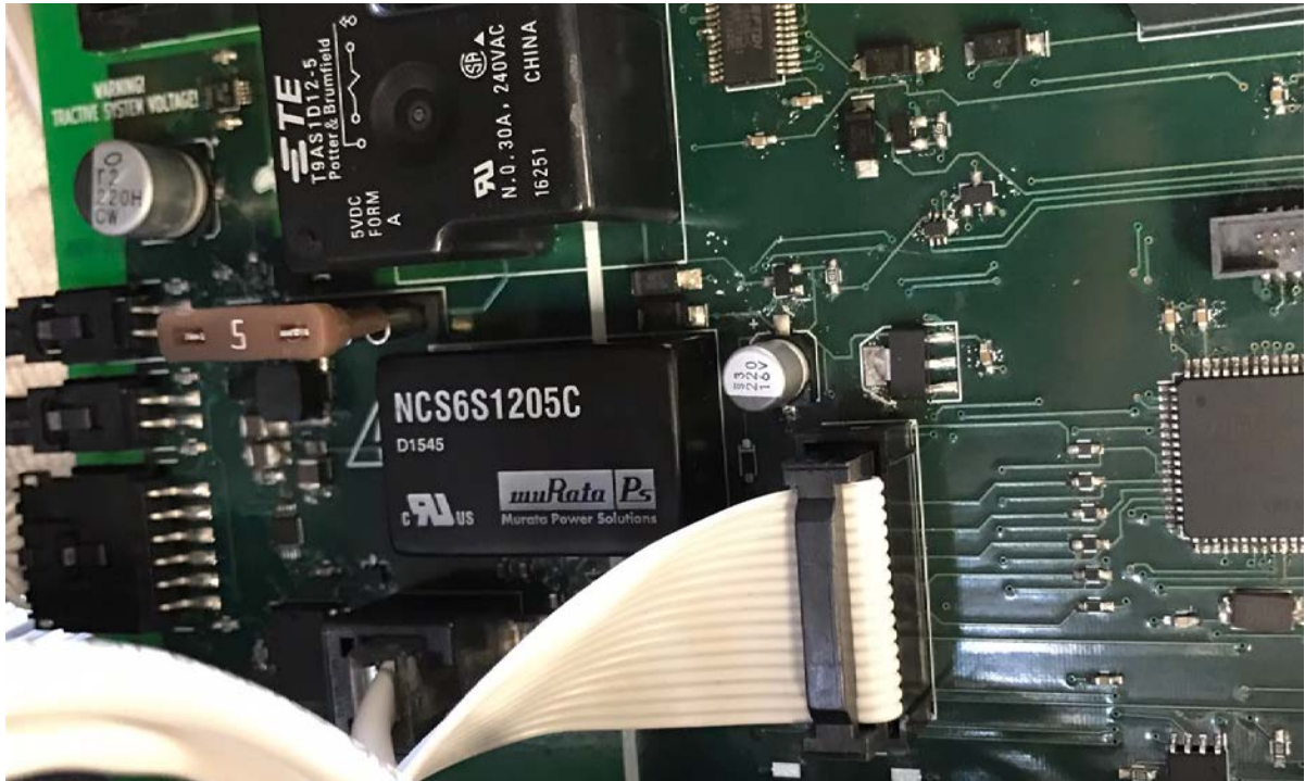
Figure 5. Installed Control Panel Connector
