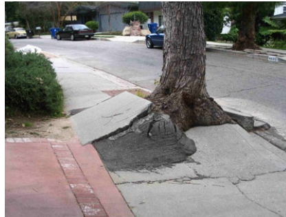
Sidewalk damage without bump-outs
