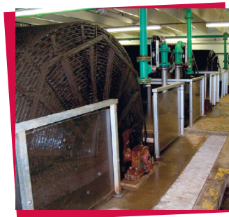
Kennebunk sewer system, Maine, USA
