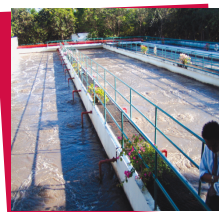
Activated sludge plant, Philippines
