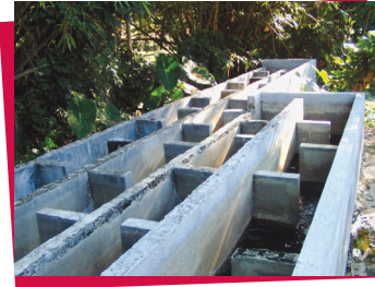
Chlorine contact basin, Muntinlupa, Philippines
