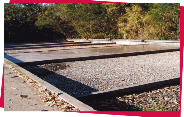
Sludge drying beds, Muntinlupa, Philippines
