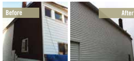
Hurricane Sandy Relief Effort - focused on assisting lower-income homeowners with repairs to their homes.
