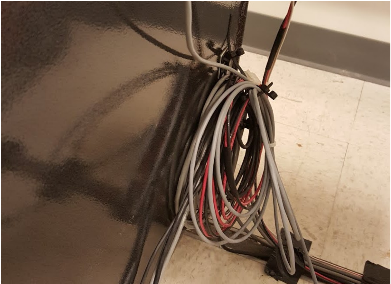
The sensor wire excess bundled before running to the Huff Box.
