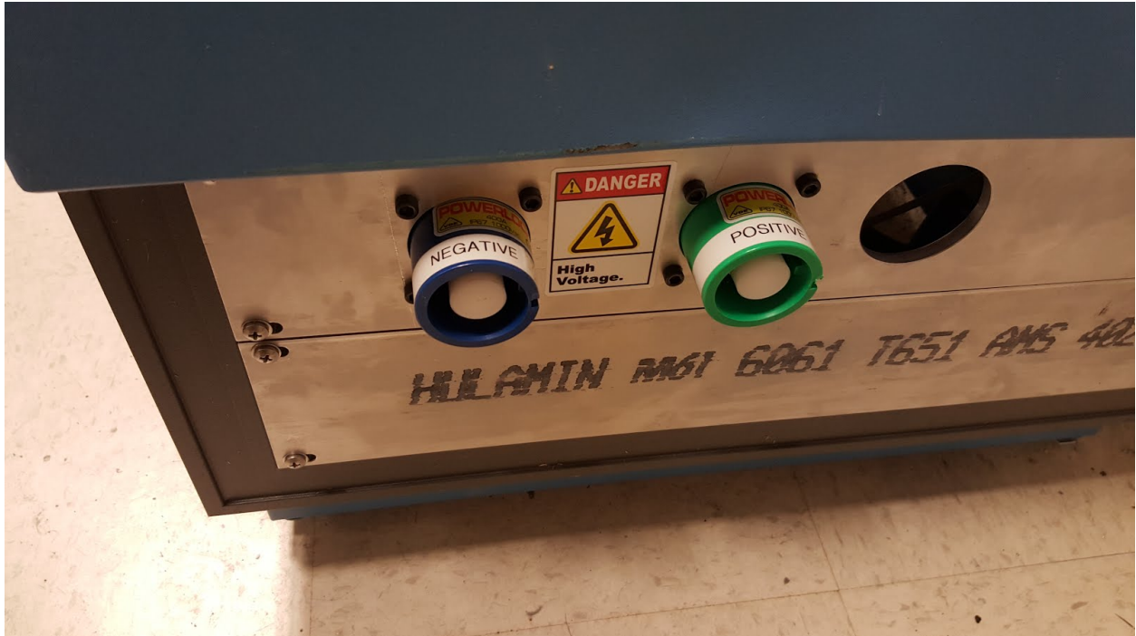
The mounting receptacles for the twist lock connectors. Each is labeled and only matching colors allow for a full connect. The hole to the right of the mounting receptacles needs to be covered over.
