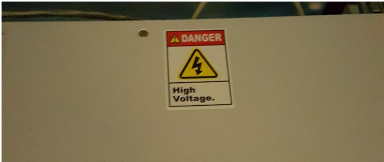
The high voltage warning sticker on the Magna Power power supply.
